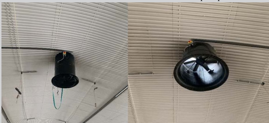
Picture 2 Fan damper open due to wind gusting.
